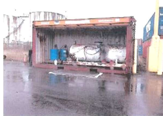
Open Storage: fuel tank
